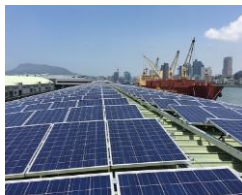
Solar Power Plants
