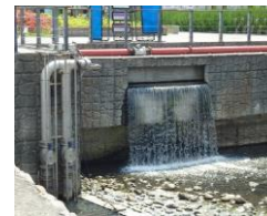
Sewage treatment and reclaimed water treatment plant
